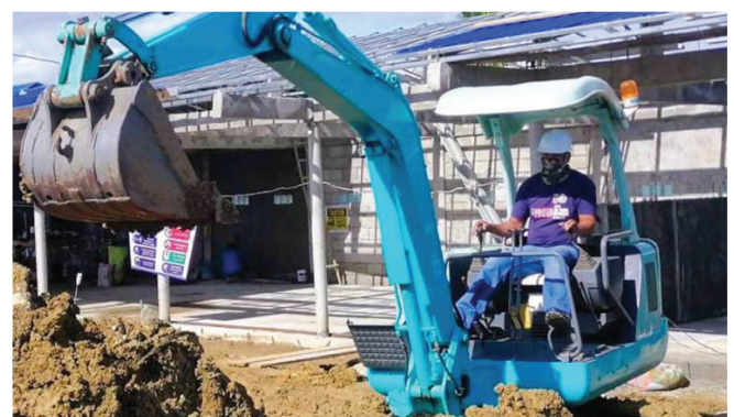
Coastal clean-up in Brgy. Taliptip as part of SMC's reclamation in Bulacan.
